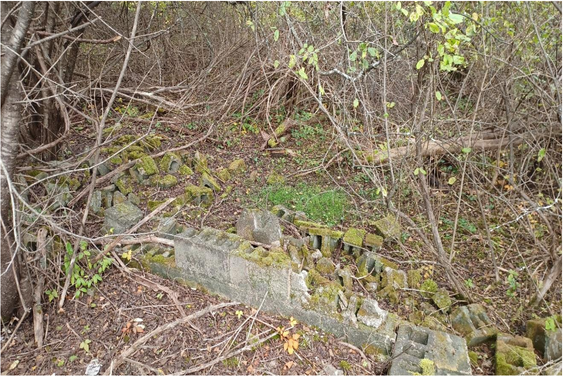
Photo 8: The barn foundation (F4) near the existing silo was constructed of concrete slabs and cinderblock. View to the northwest.
