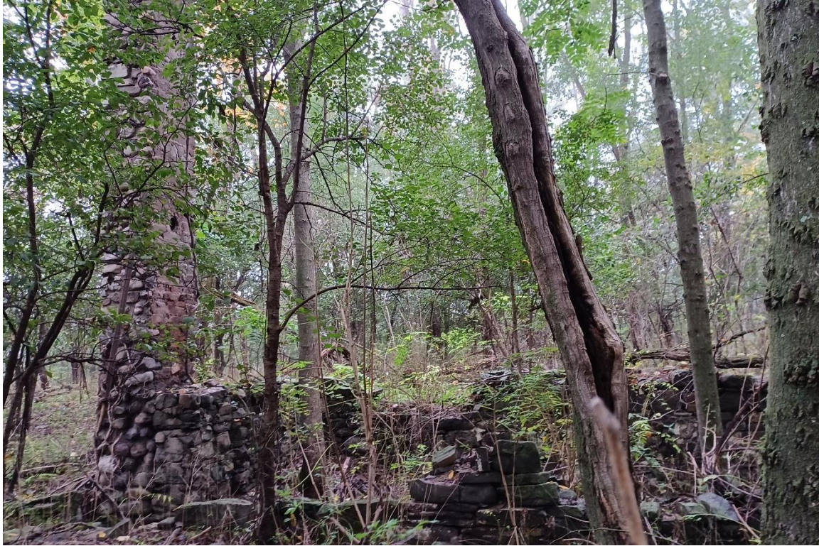
Photo 23: The foundation for the residential structure (F2) features modern concrete and a gutter on the outside of the chimney. View to the southwest.
