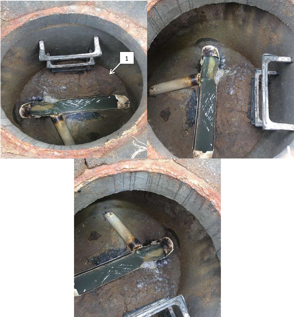
Minor damage [1] Minor debris, no invert
