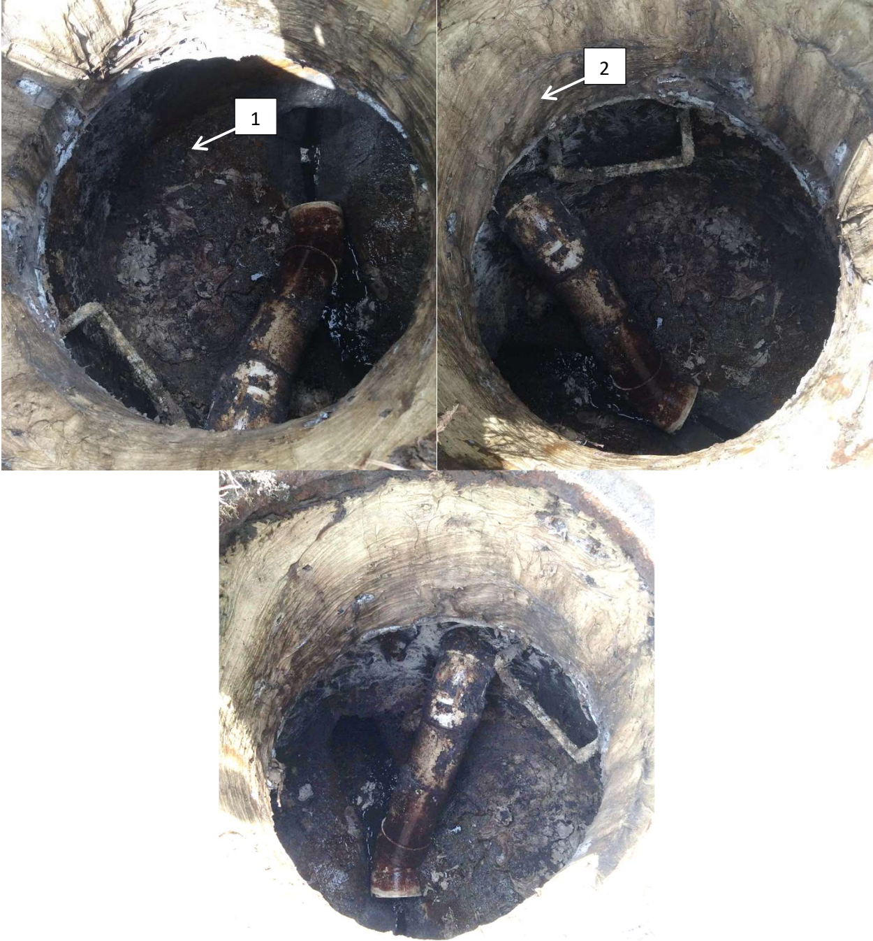
A lot of damage [1] Grease and other debris buildup [2] Concrete erosion cracks in water stop
