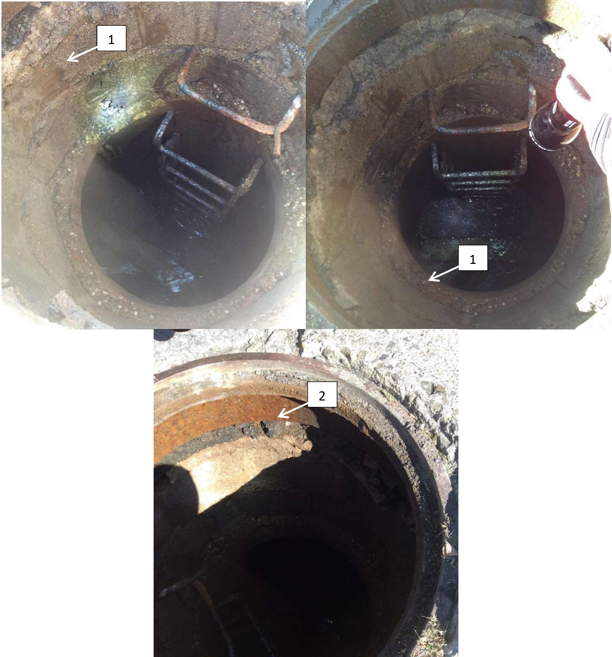
A lot of damage [1] Concrete erosion [2] Rust
