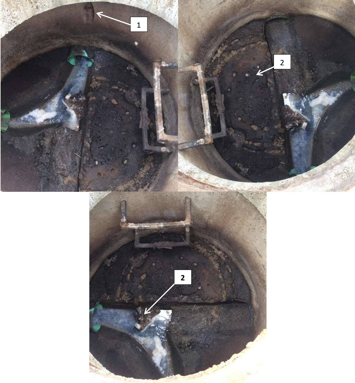
Minor damage [1] Rebar Exposure [2] Debris buildup within invert
