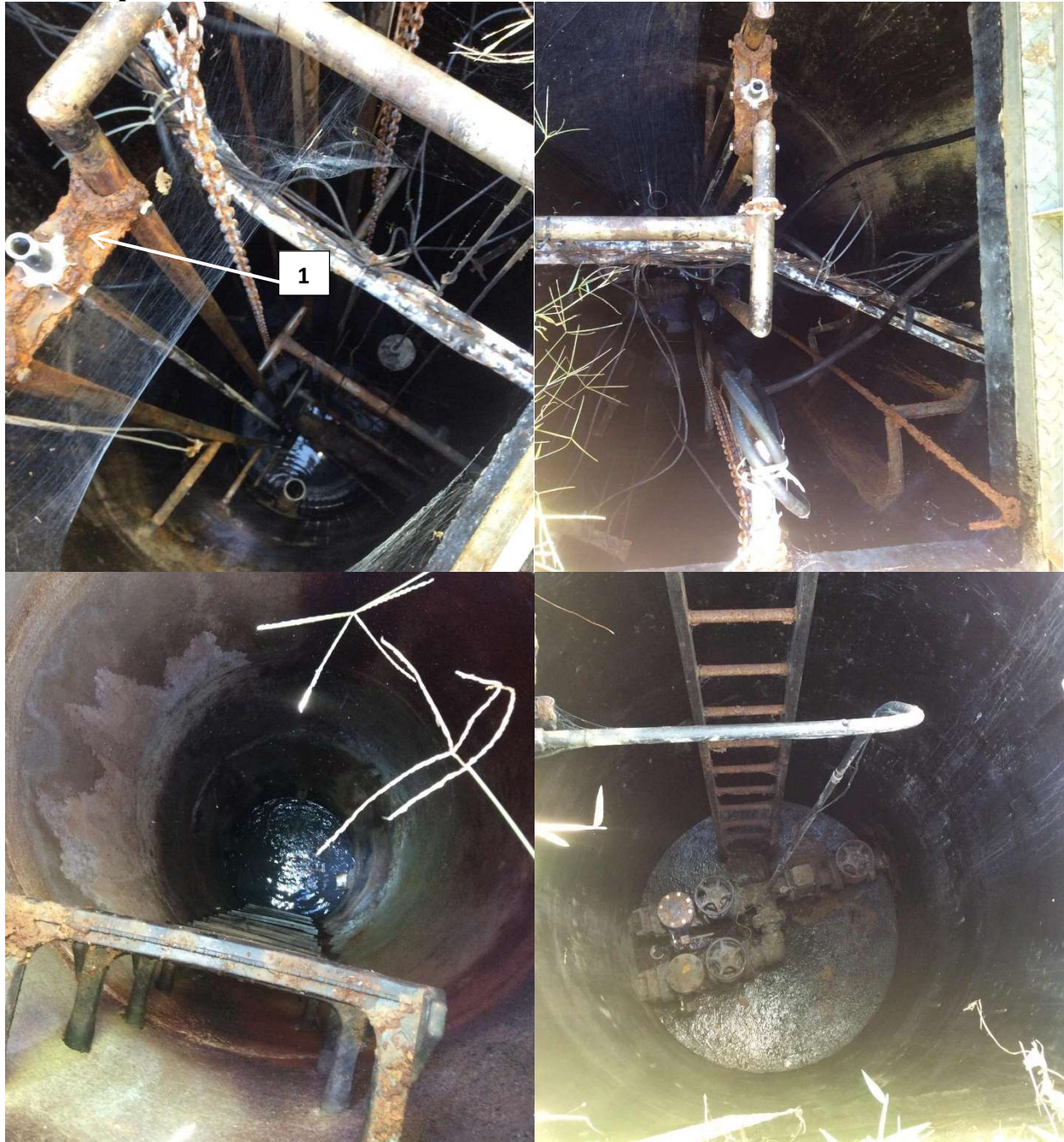
Little to no damage [1] Top slide rail support shows corrosion
