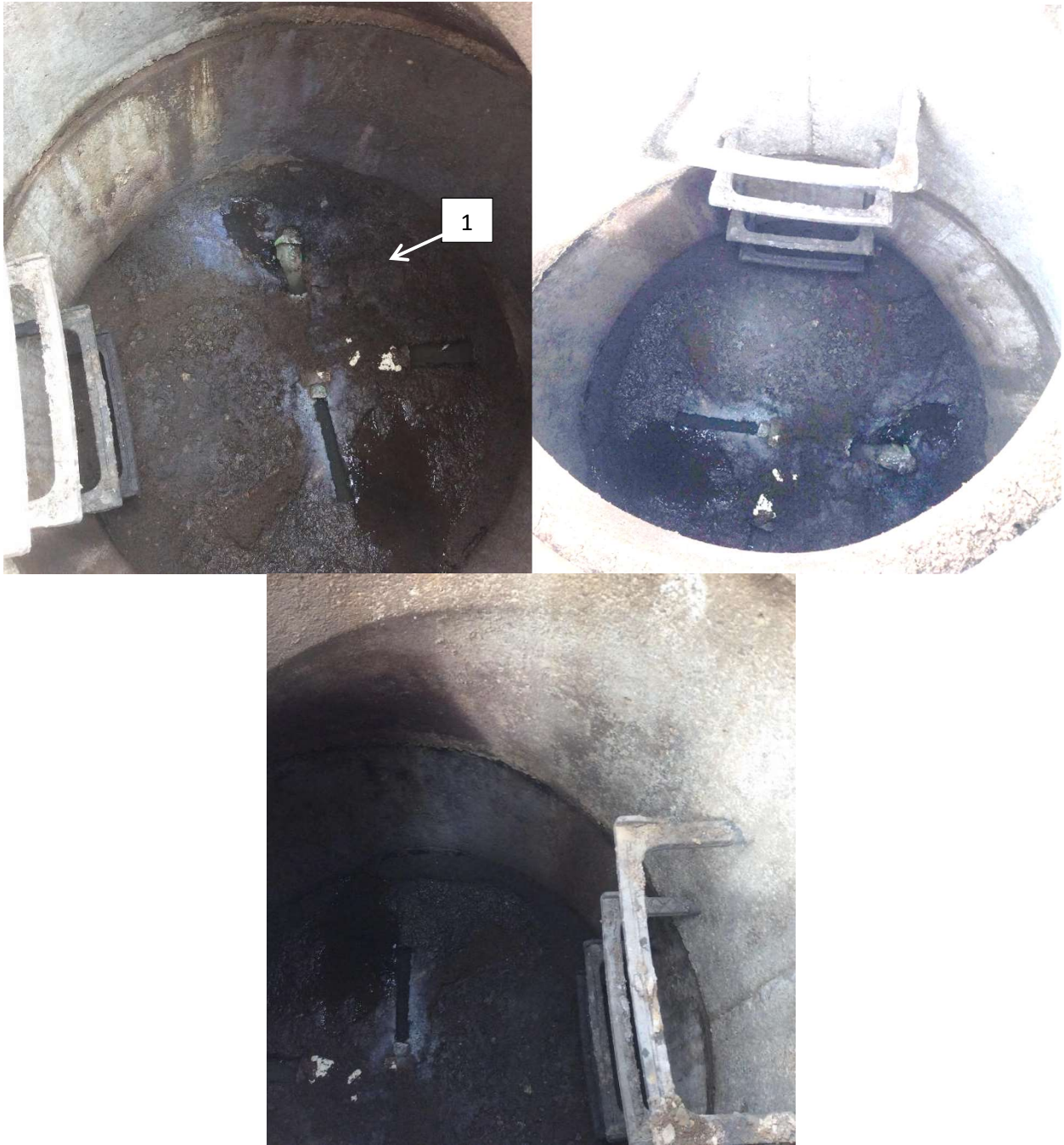
Minor to no damage [1] Standing water and debris on bottom Appears to be sludge from downstream backups.
