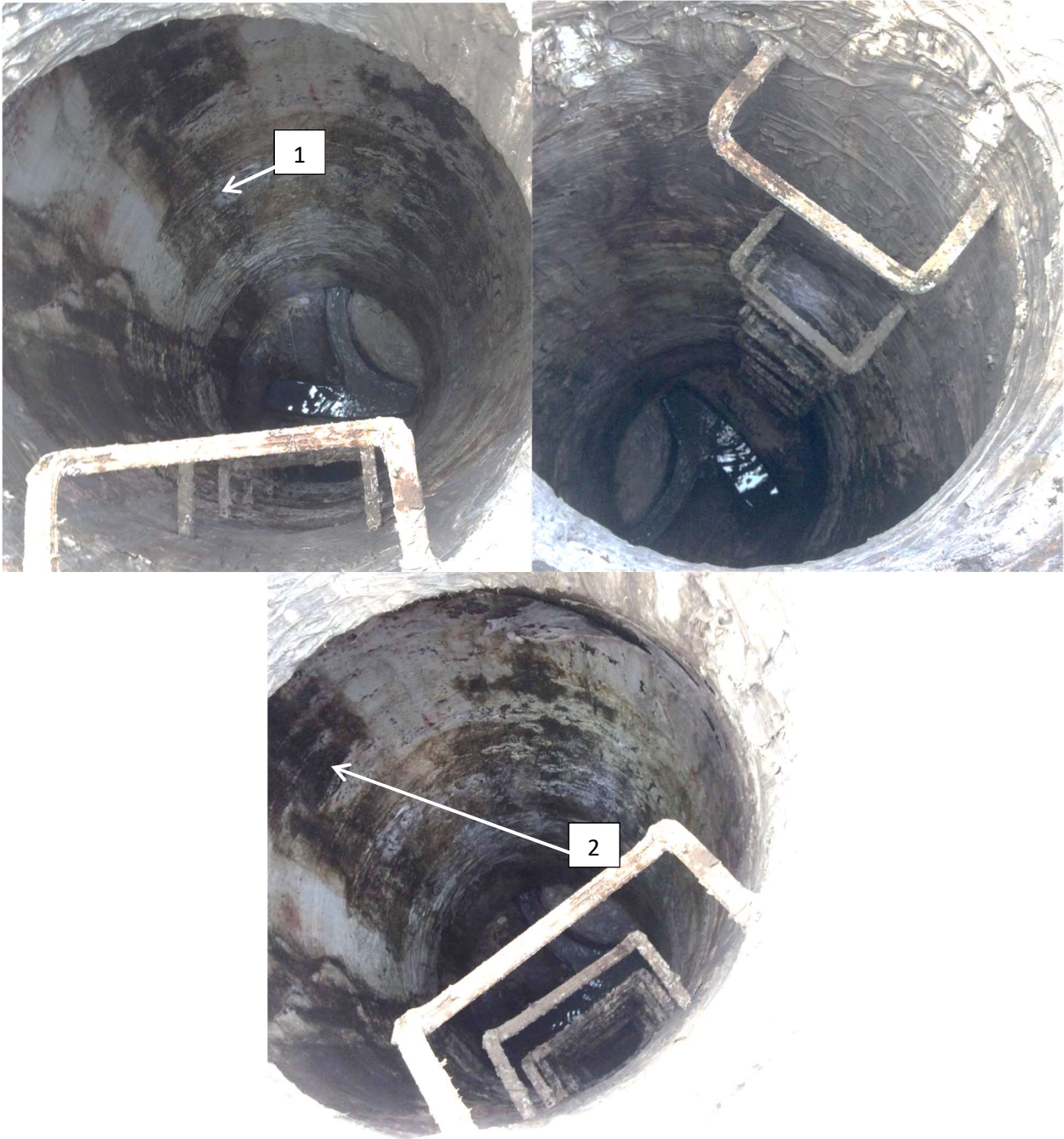
Some damage [1] MH coated with water stop coating [2] Water Stop discolored
