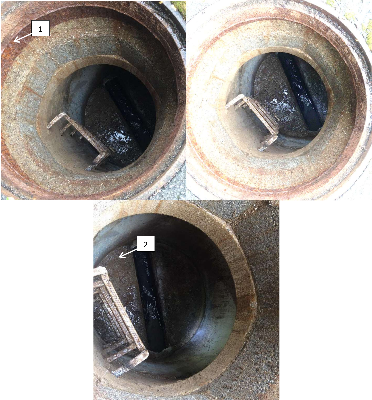
Little to no damage [1] Rust [2] Standing water & debris on bench
