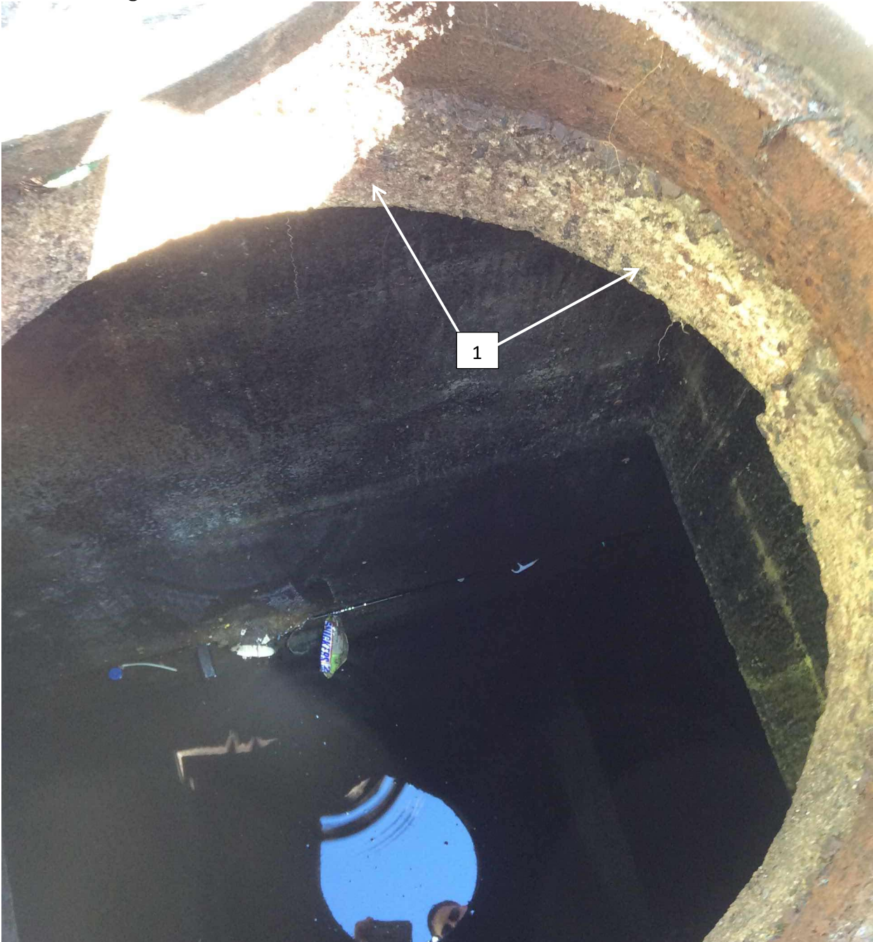
Minor to no damage [1] Concrete erosion
