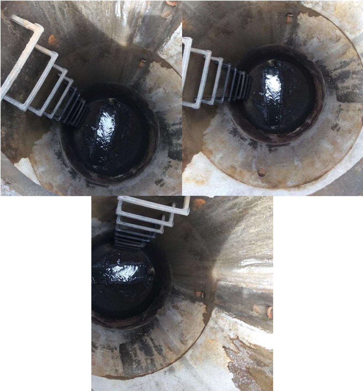
Minor to no damage
