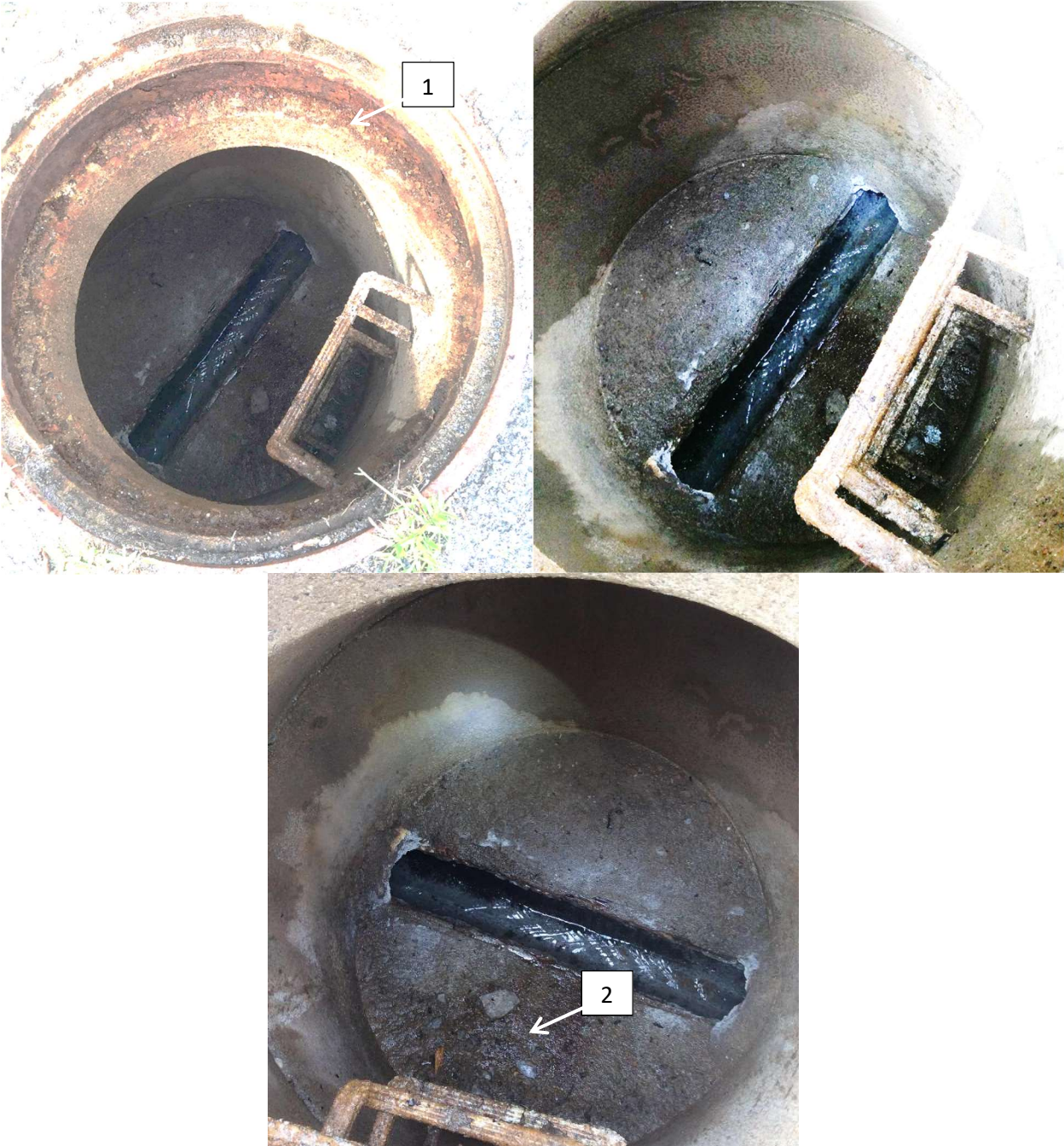
Little to no damage [1] Rust [2] Debris on bench, bench is wet
