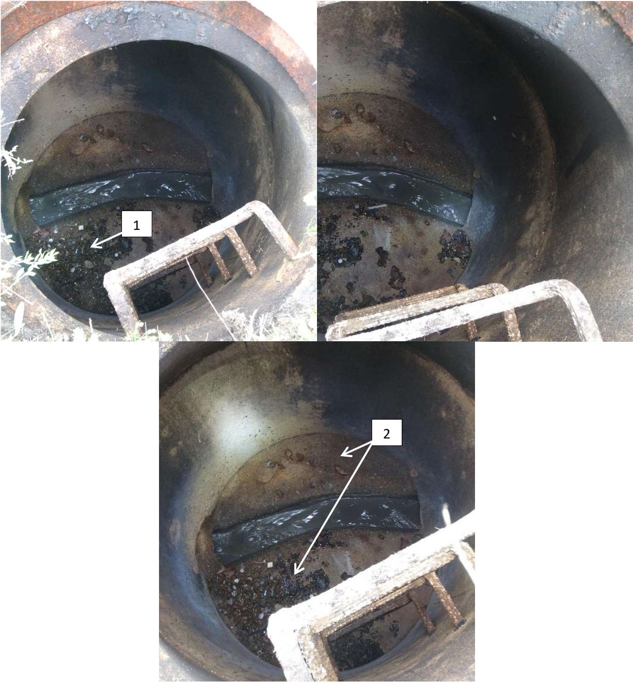
Some damage [1] Gravel on bench [2] Concrete erosion & debris on the bench
