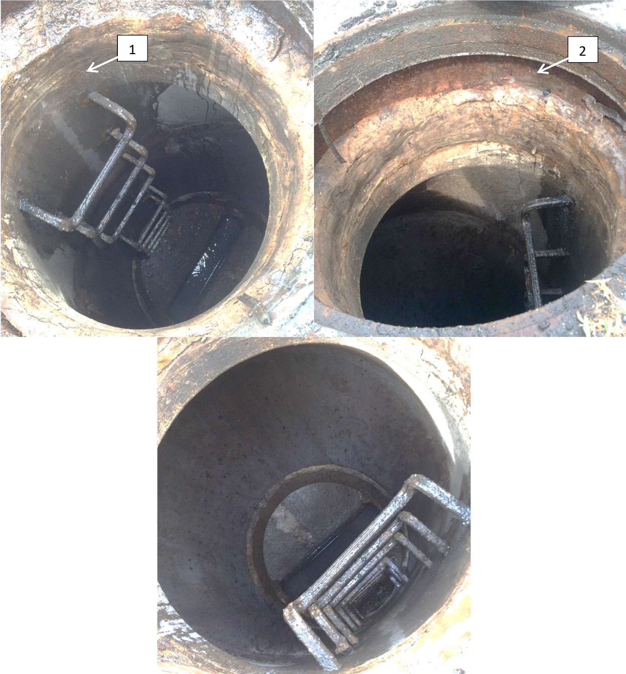
Some damage [1] Mortar under ring not tight [2] Rust
