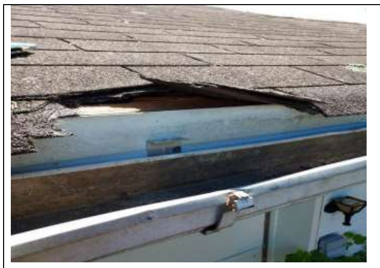
View of 483 Beaver Dam Road – Roof Shingle
