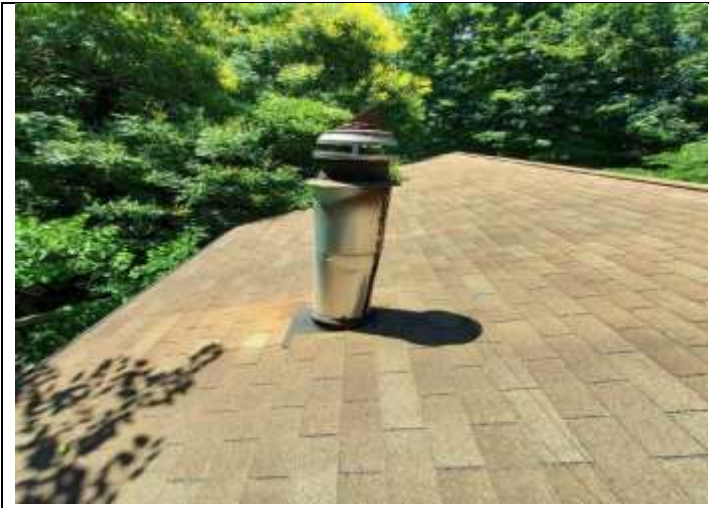
33. View of 475 Beaver Dam Road – ACM Vent Flashing
