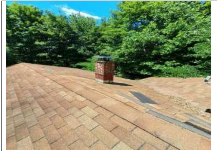
34. View of 475 Beaver Dam Road – ACM Chimney Flashing
