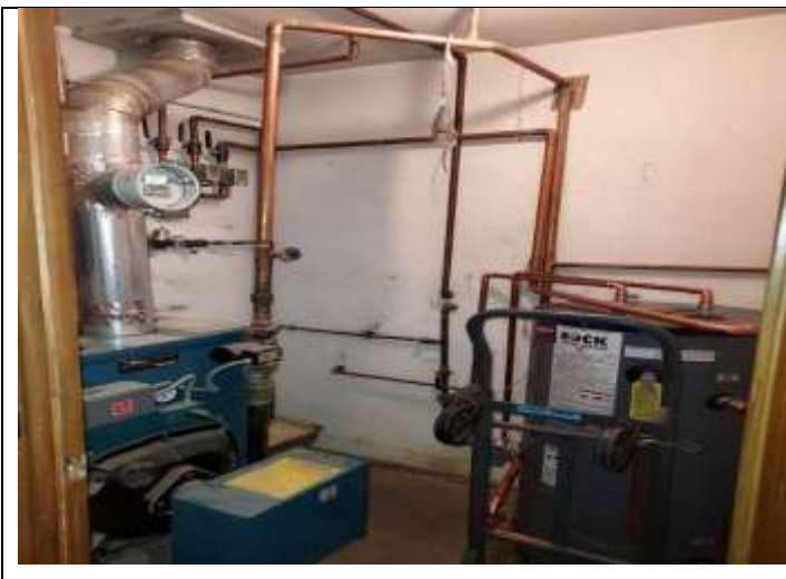
17. View of 497 Beaver Dam Road – Furnace
