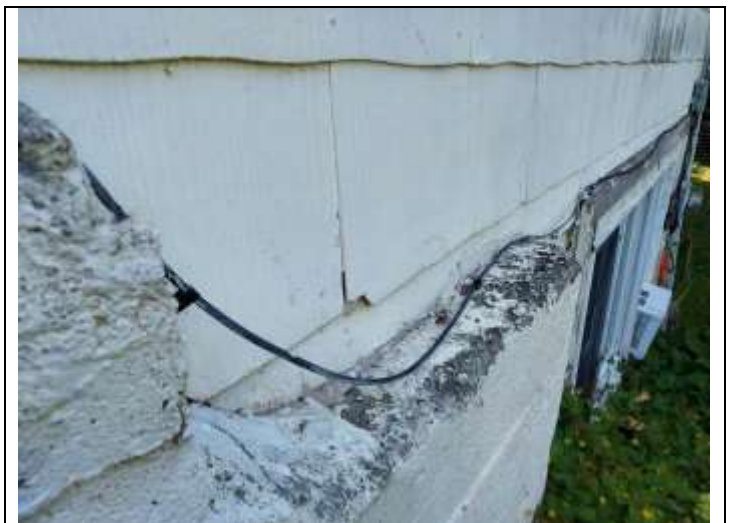
22. View of 497 Beaver Dam Road – ACM Transite Shingles
