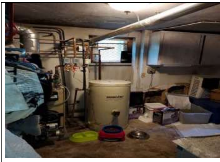
29. View of 497 Beaver Dam Road – Basement Furnace and Hot Water Heater
